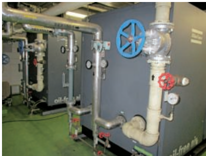
Compressor before replacement
