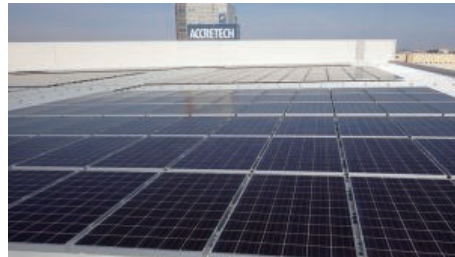
Solar panels at Hachioji Plant No. 6
