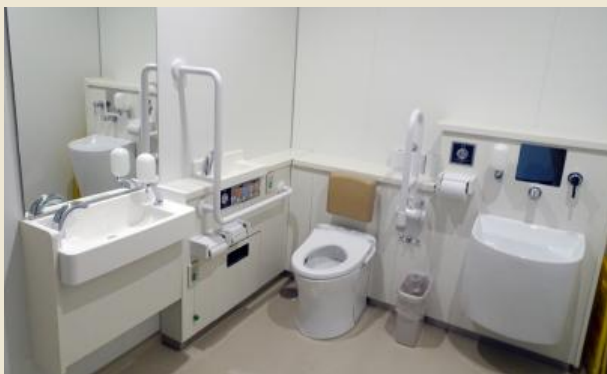
Multi-purpose Restroom of the No. 6 Plant in Hachioji
