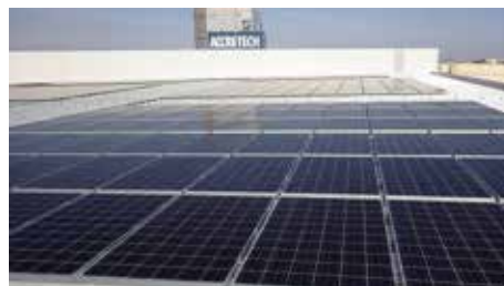
Solar panels at Hachioji Plant No. 6
